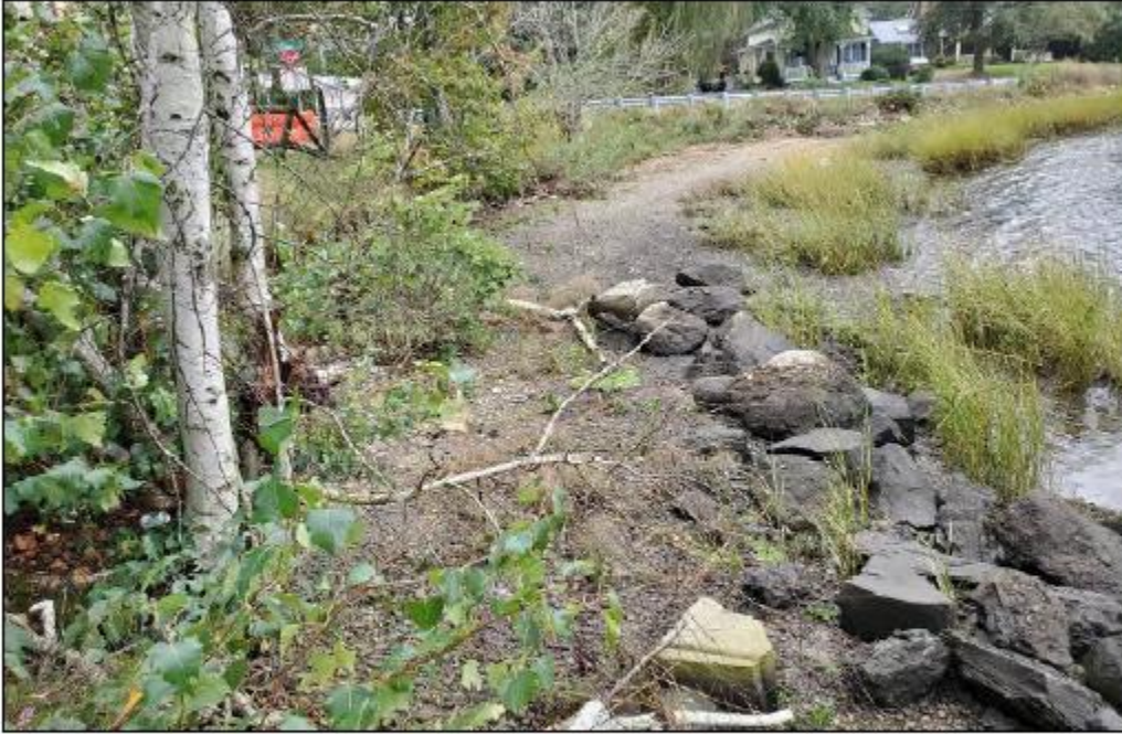
Photo No. 13: North embankment at east abutment looking east near Sowams Road
