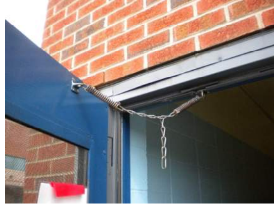
Photo A8: Door closer missing.
