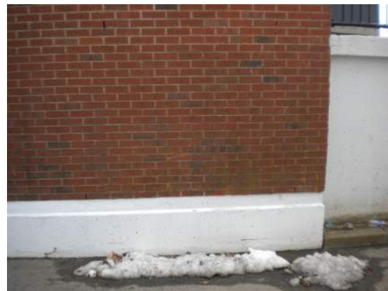
Photo A3: Green growth on bricks.
