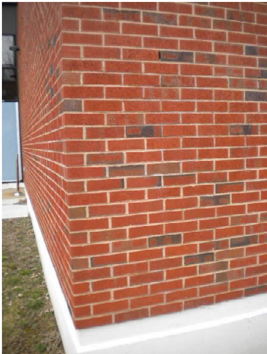
Photo A19: Vertical crack.
