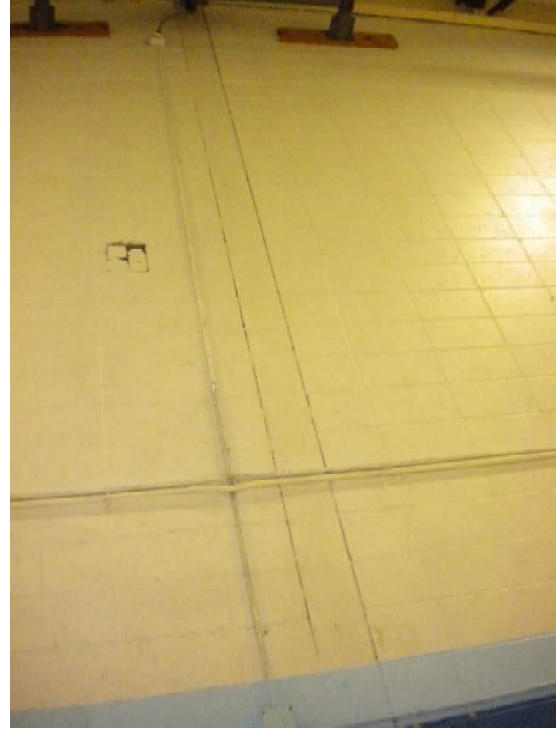
Photo B14: Damaged CMU.
