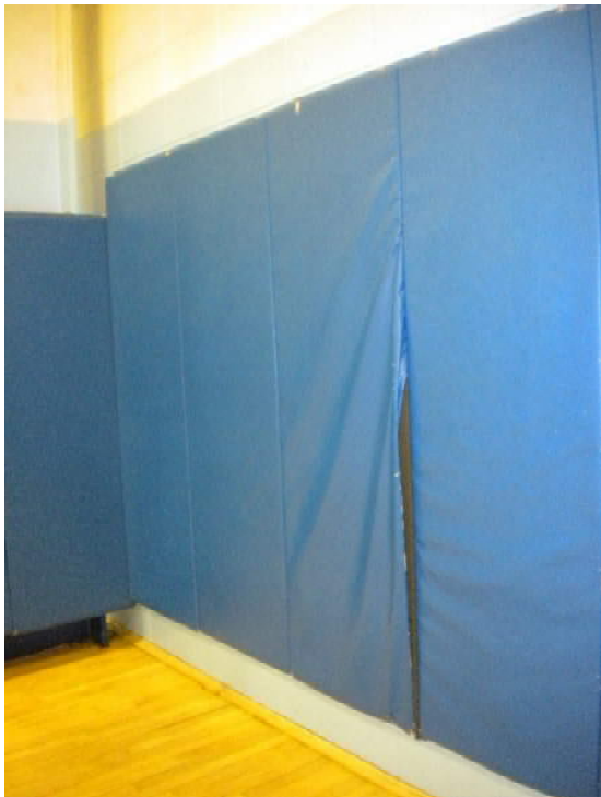
Photo B11: Damaged existing padding.
