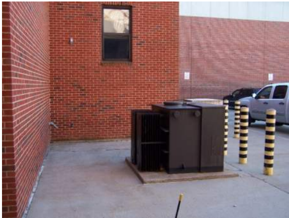
Photo A1: Transformer.
