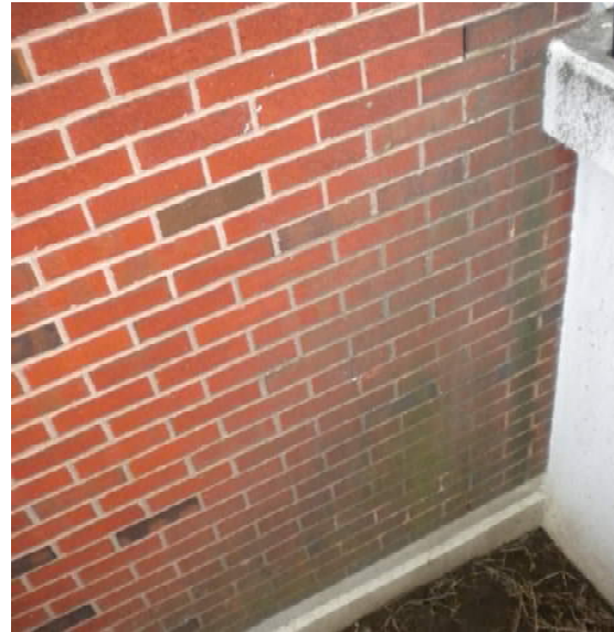
Photo A3: Green growth on bricks.
