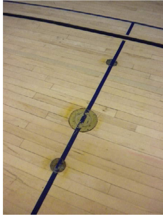
Photo B12: Metal sleeves with cover plates.
