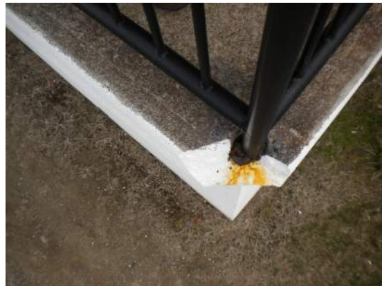
Photo A11: Concrete missing at railing sleeve.
