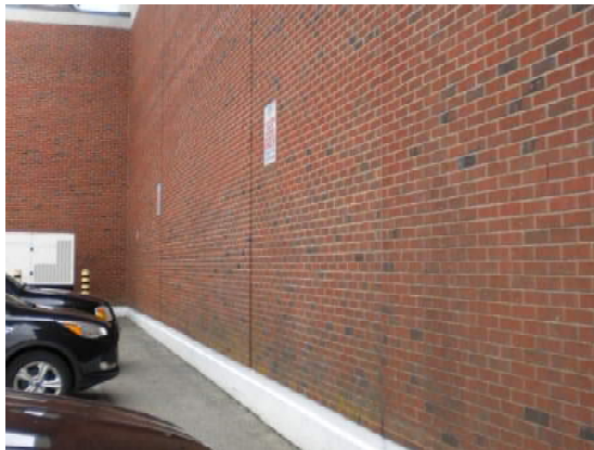
Photo A3: Green growth on bricks.
