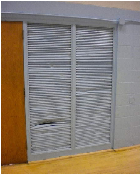
Photo B1: Damaged louvers.
