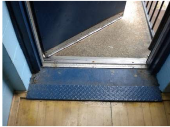
Photo A9: 2 nd diamond plate threshold.
