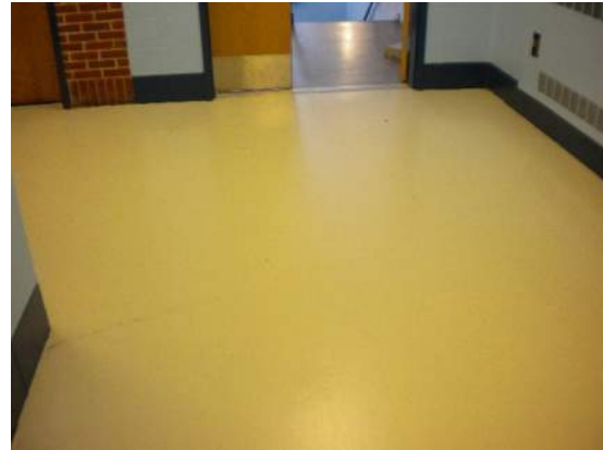
Photo C5: Crack in floor, Southwest corridor
