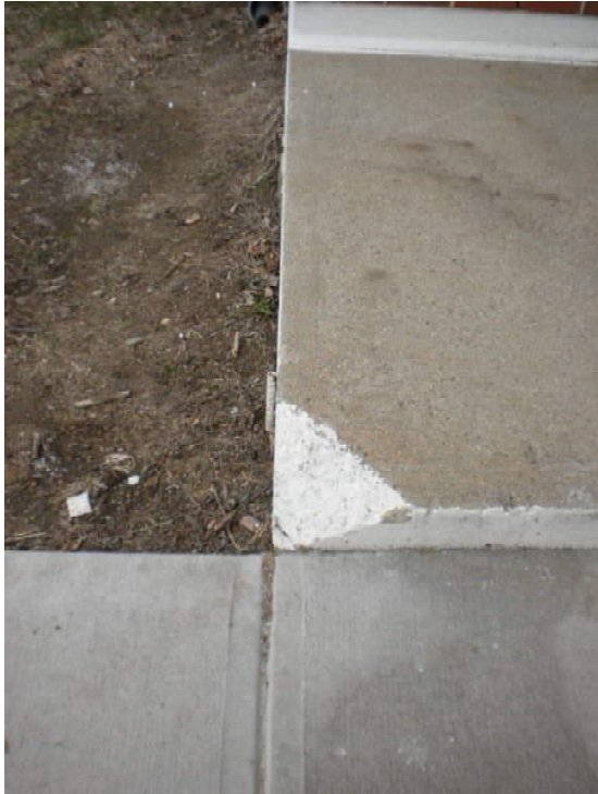
Photo A17: Concrete Corner missing.
