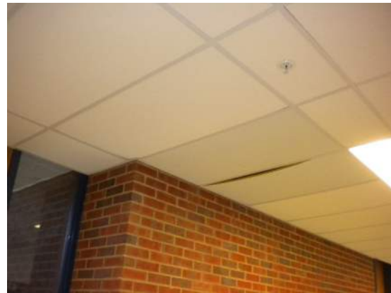
Photo C12: Sagging ceiling tile
