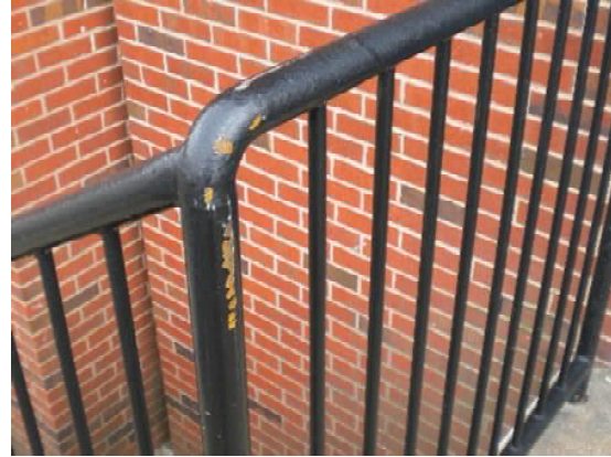
Photo A13: Chipped paint on railing.
