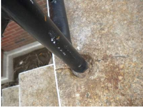
Photo A12: Crack in concrete at sleeve
