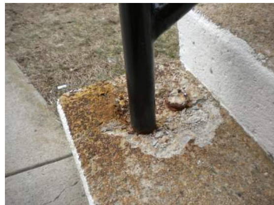
Photo A6: Rust / cracking / railing disconnected.
