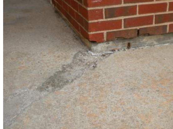
Photo A2: Chipped bricks & walkway.
