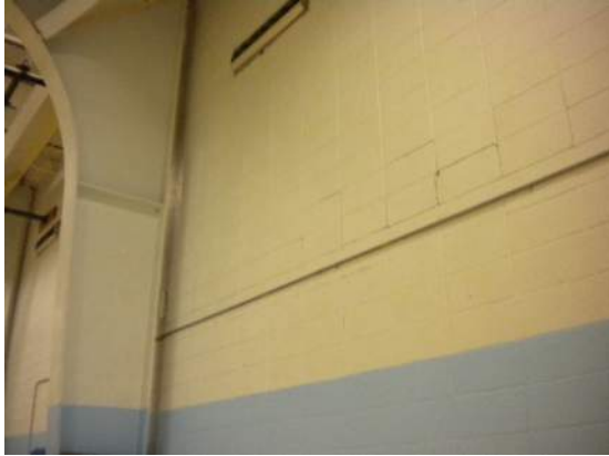
Photo B16: Cracking in CMU mortar
