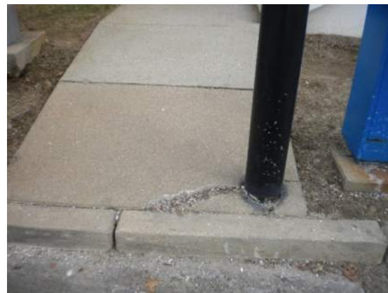
Photo A15: concrete deterioration at bollard.
