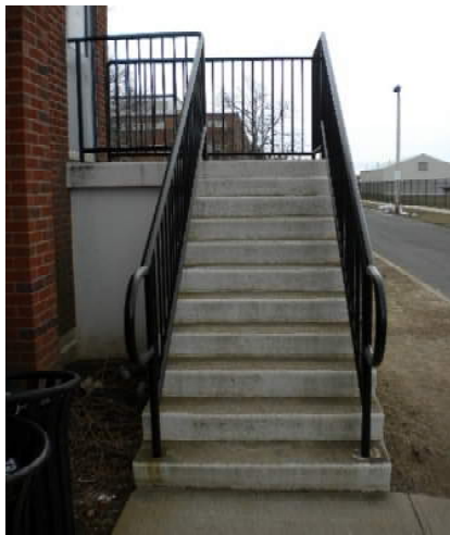
Photo A10: Right railing is loose
