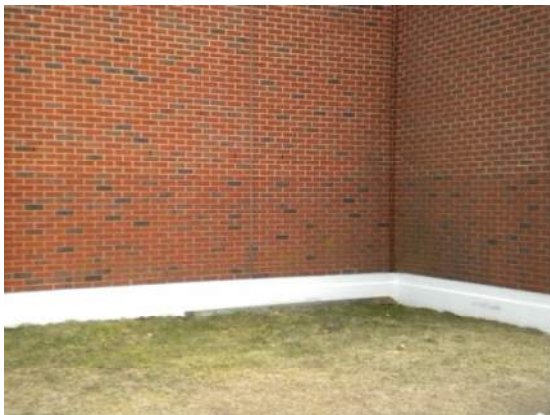
Photo A3: Green growth on bricks.
