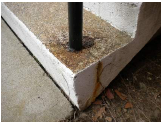
Photo A5: Rust / cracking at stair.
