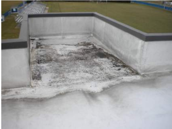
Photo A1: Standing water @ roof.
