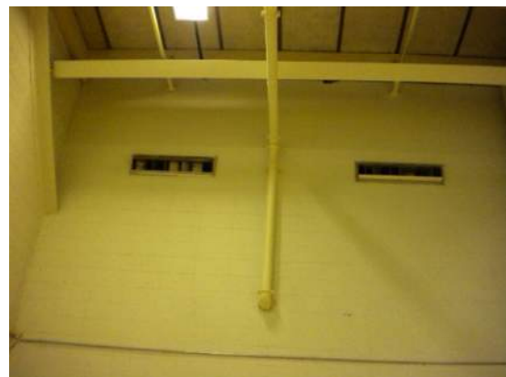
Photo B8: Existing HVAC Supply grilles.
