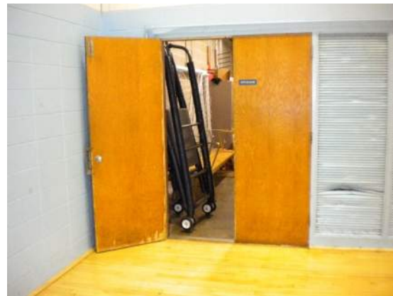
Photo B2: Damaged doors.
