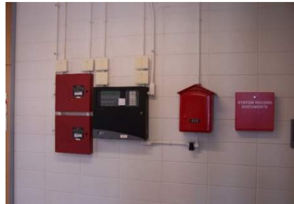
Photo D1: Fire Alarm System.
