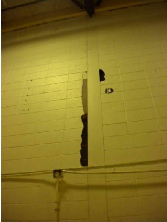
Photo B13: Damaged CMU and conduit.
