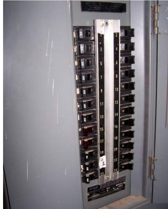
Photo A1: Typical electrical panel.
