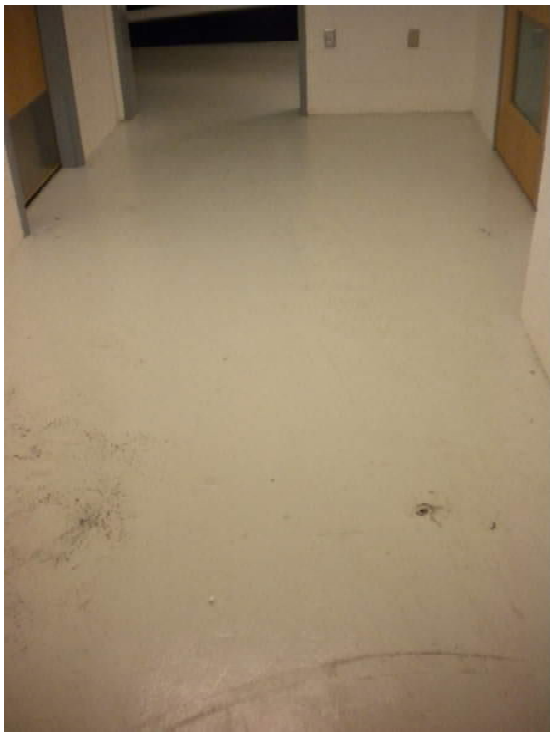
Photo C5: Chipped floor finish, Elevator vestibule
