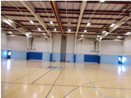
Photo B15: Moveable partition enclosure
