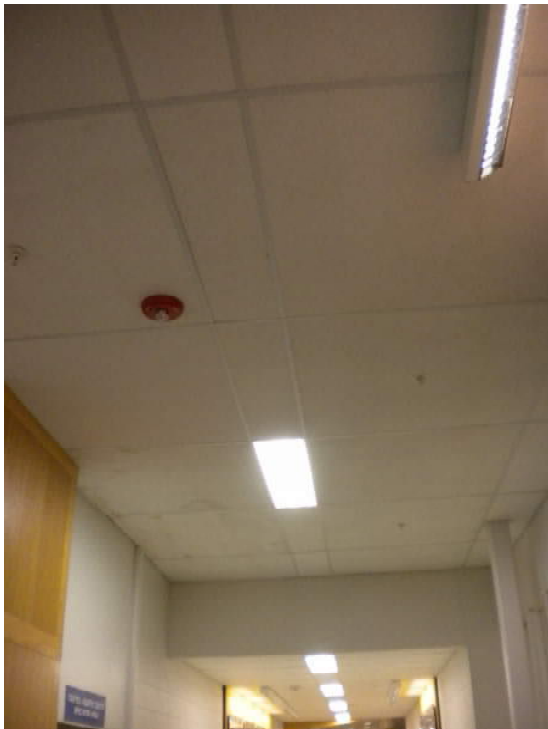
Photo C7: Water damage to ceiling tiles
