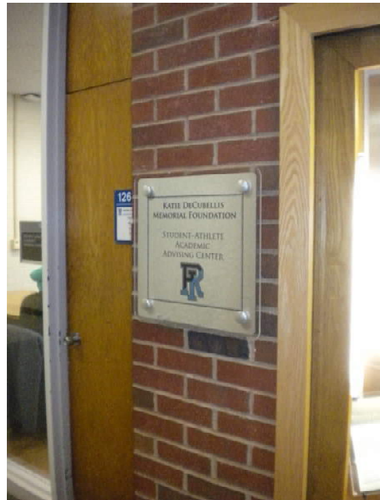
Photo C8: Chipped paint on door frame
