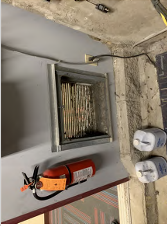
Machine Room Exterior Vent
