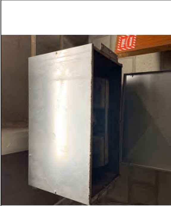
Machine Room HVAC System
