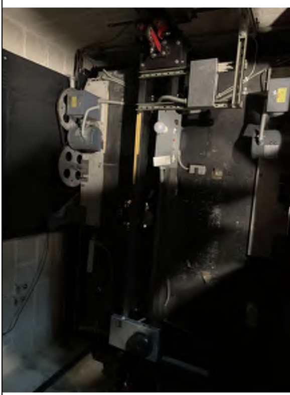
Top of Elevator Cab – Dual Door Operators
