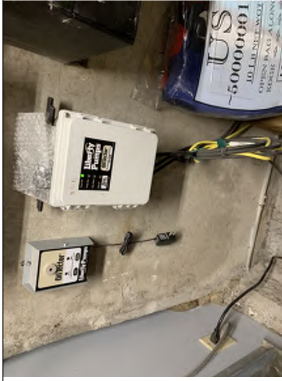
Pit Area Sump Pump Power Unit
