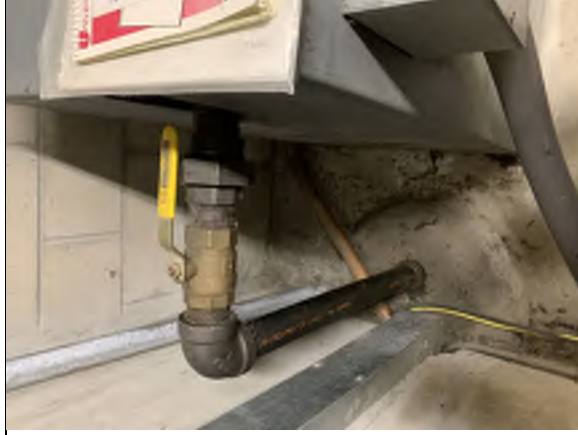
Hydraulic Piping System and Valves
