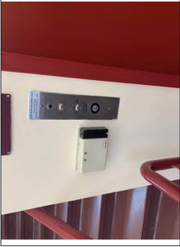
Hall Call Station with Keyed Tenant Access
