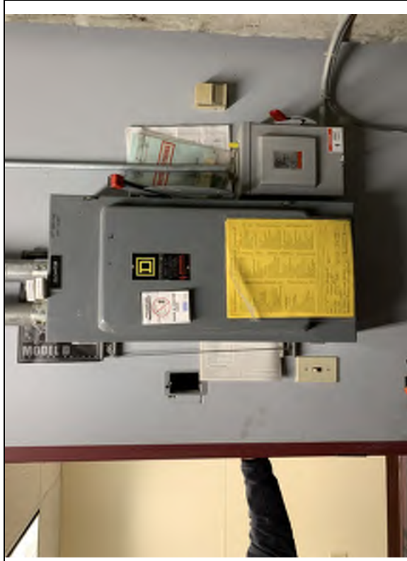
Mainline Disconnect and Cab Lights
