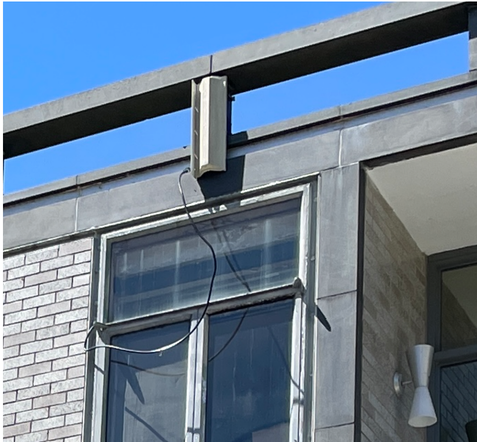
Antenna at West side of bldg:
