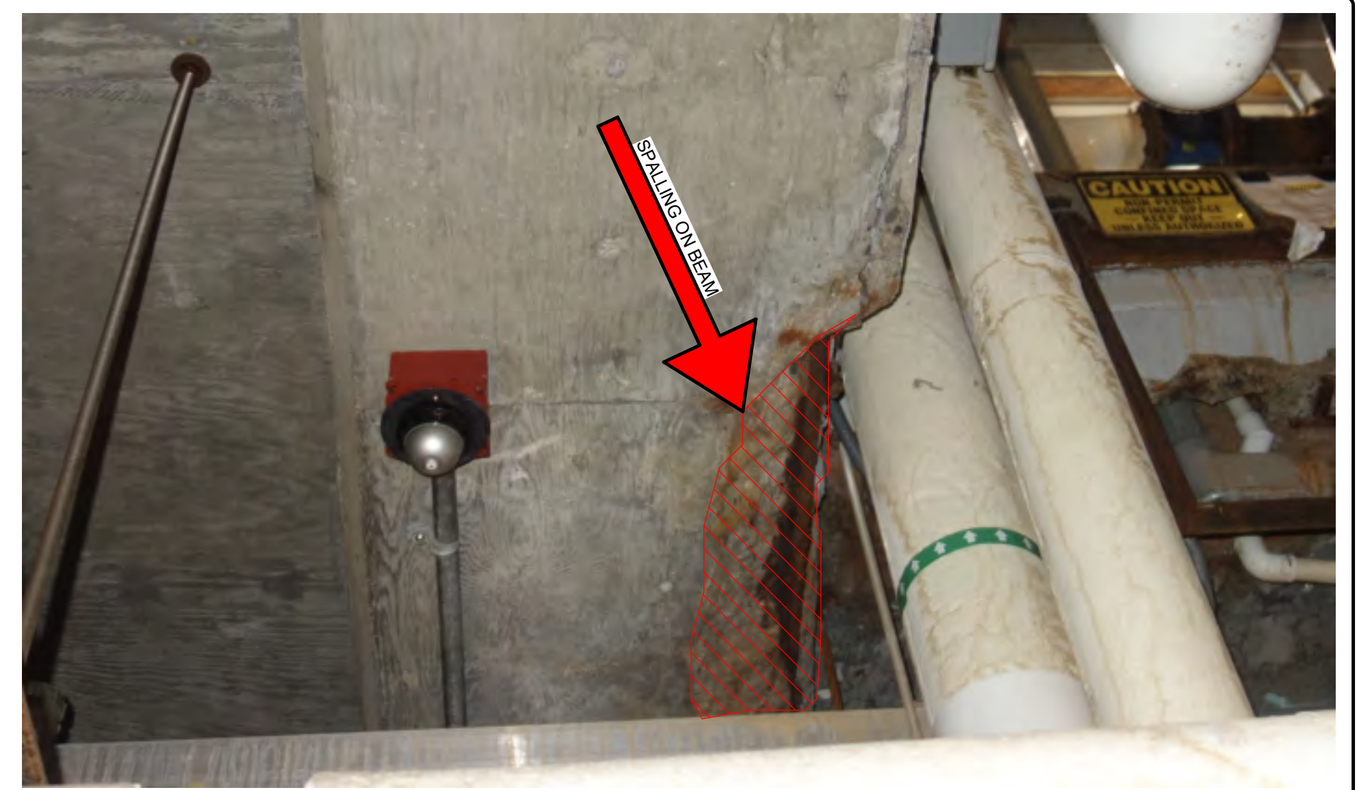
B2 PHOTOGRAPH OF DEFICIENCY (LOOKING UP) - DETERIORATED CONC. BEAM CORNER AND VERT. FACE B DEFICIENCY B - BEAM CRACK & SPALLING NO SCALE
