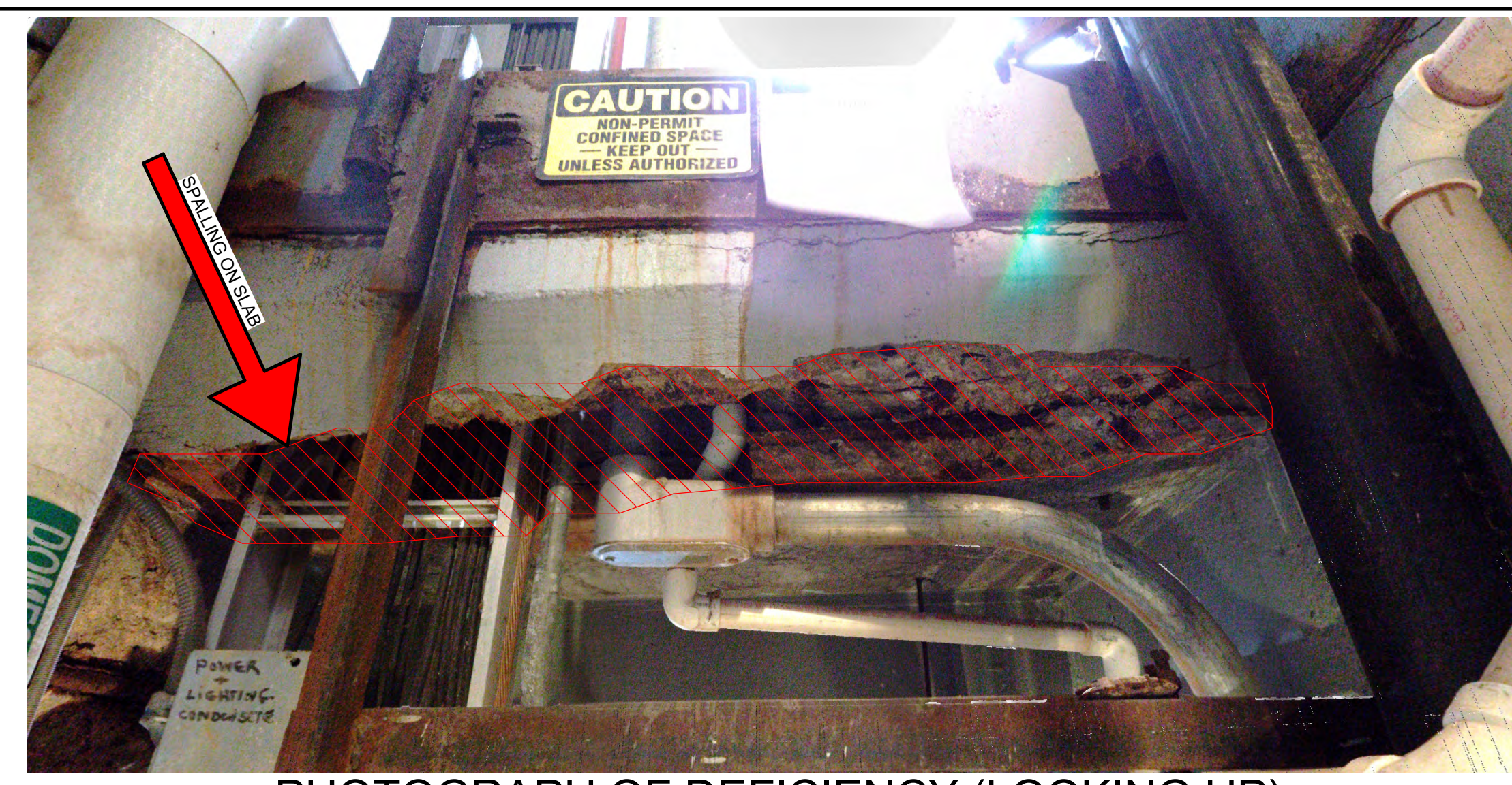
C1 PHOTOGRAPH OF DEFICIENCY (LOOKING UP) - DETERIORATED DECK EDGE C DEFICIENCY C - FAILED SLAB DEMOLITION NO SCALE
