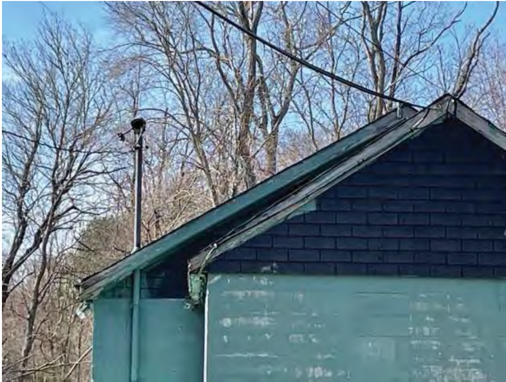
Photo 4 – Electrical Services to URI Radio Tower Control Room
